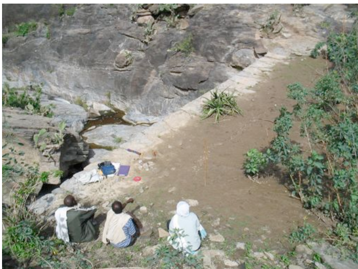
Illustration 40: Up view on the Ubuktole Ela check dam, showing the running brook coming out of the check dam’s bottom; August 2003
